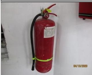
Photo of fire safety equipment Fire Extinguisher.JPG
