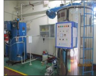
External photo(s) of the production unit(s) Boiler.JPG
