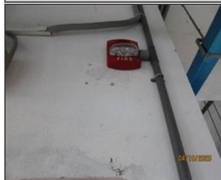
Photo of fire safety equipment Fire alarm.JPG
