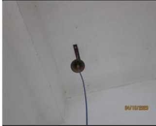
Photo of fire safety equipment Gong bell.JPG
