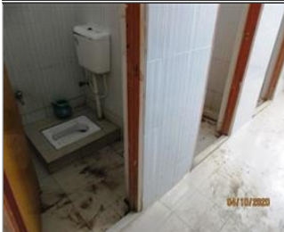
Photo of non-conformity Finding 7.22 Workers toilets were not clean and tidy.JPG
