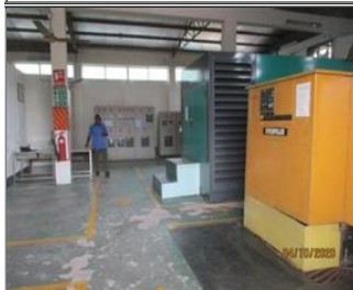
External photo(s) of the production unit(s) Generator.JPG
